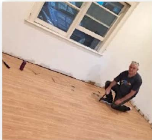
The floor in one of the main bedrooms needed to be replaced .
